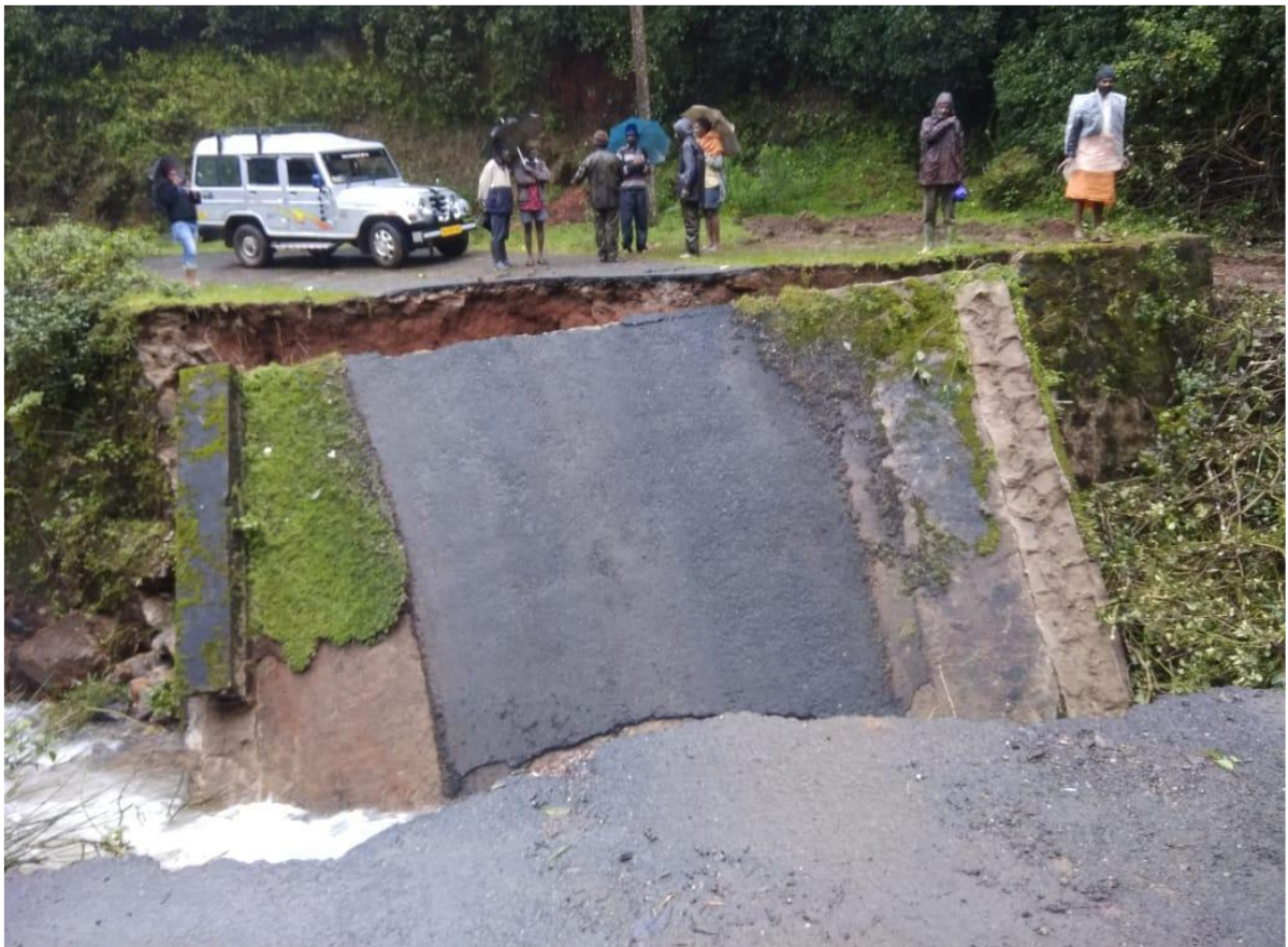
Figure: 5.1 - Damaged road at TR Bazaar Terrace Estate Road
