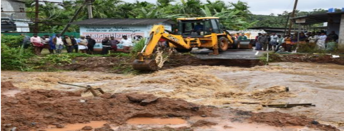
Figure 5.2 - Manguli Bridge in Gudalur Taluk damaged due to heavy rainfall
