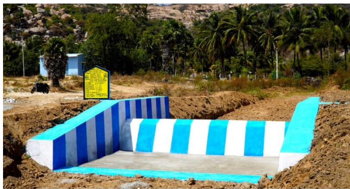
NAME OF THE DISTRICT : KRISHNAGIRI NAME OF THE WORK : CONSTRUCTION OF CC CHECK DAM AT B G PUDHUR NAME OF THE BLOCK : KRISHNAGIRI NAME OF THE SCHEME : MGNREGS NAME OF THE HABITATION : B G PUDHUR ESTIMATE AMOUNT : 5.420 LAKHS NAME OF THE PANCHAYAT : KALLUKURUKKI
