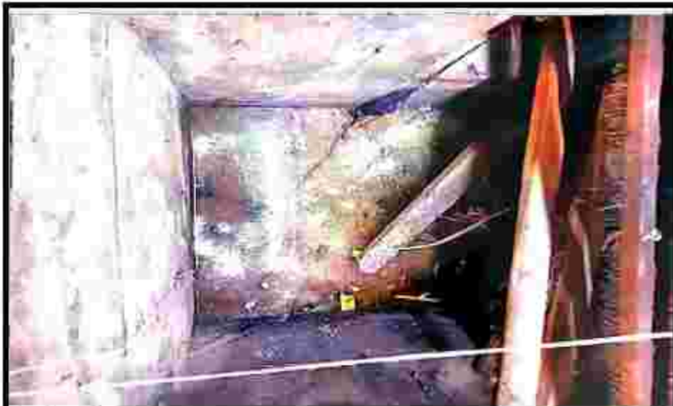
Oozing of water in pitloom in Mannarpoluru (V), Sullurupeta Municipality
